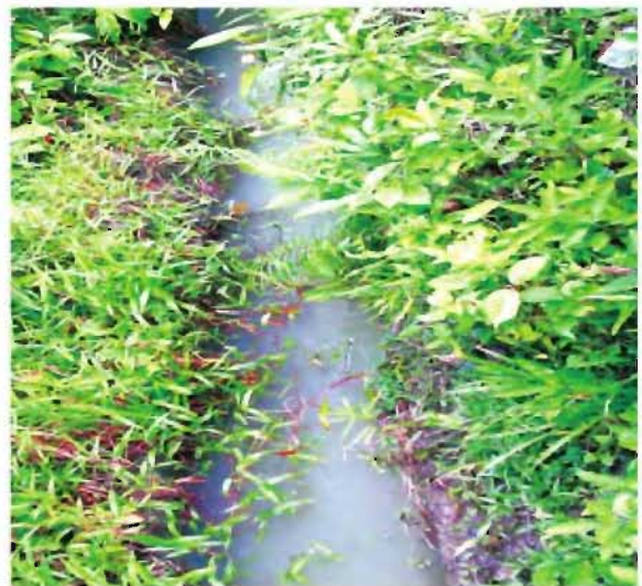
Rain water drainage on Ring road
